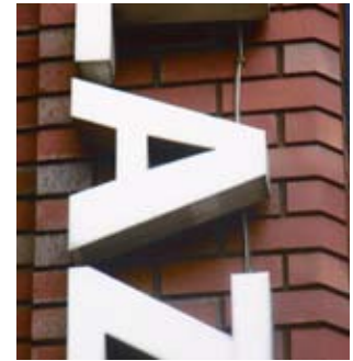
Series wiring visible between each letter, on brickwork
